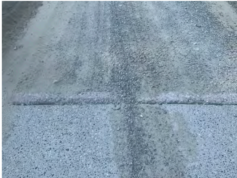
Deck, ballast wall. Rebar showing. Right bank
